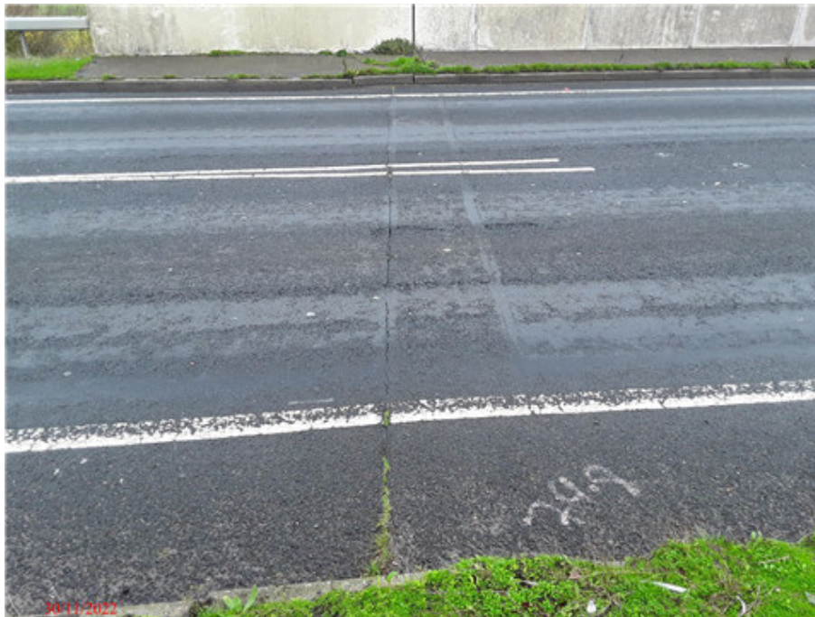
Span 3 - West Carriageway Cracks to APJ edges
