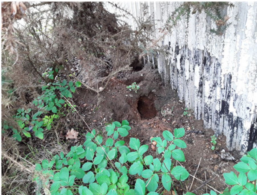
Span 1 - South East Embankment Animal habitat undermining elements
