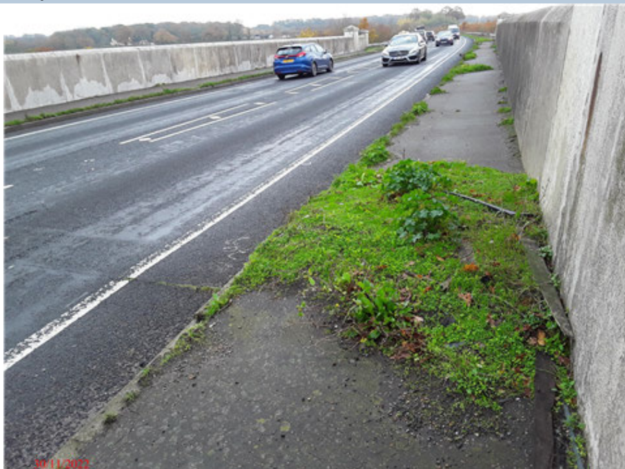
Span 3 - West Footway Vegetation build up to footway front edge and joints.
