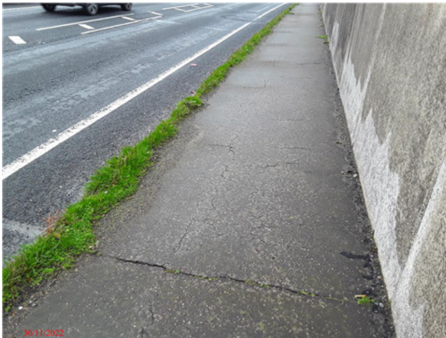
Span 2 - East Footway Minor cracks to footway
