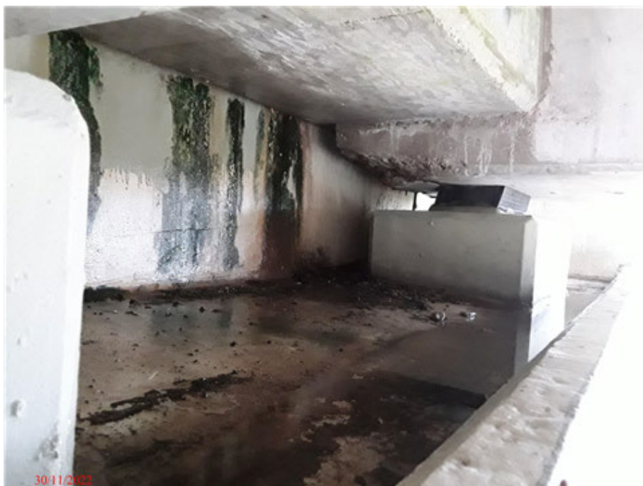
Span 1 - South West Bearing Shelf Water pooling on bearing shelf.
