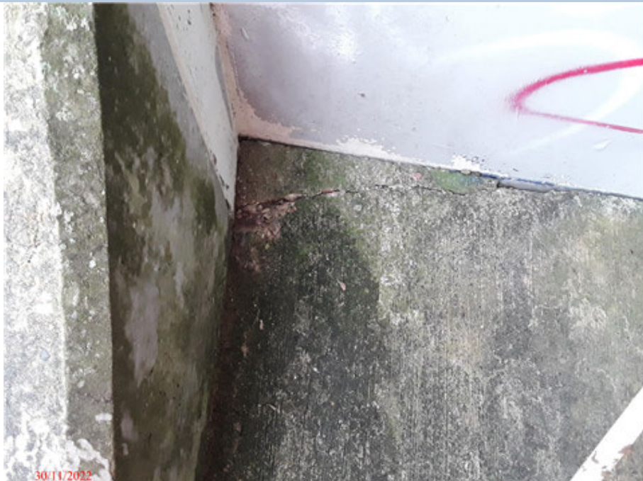
Span 1 - South East Abutment Concrete crack
