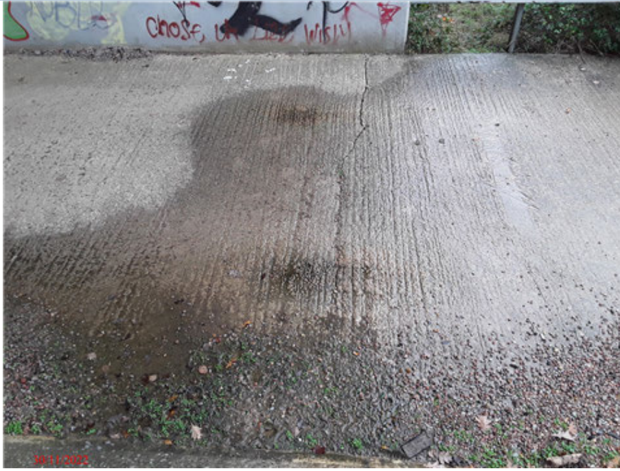
Span 1 - South East Substructure Carriageway Concrete crack
