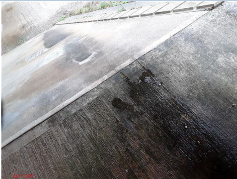
Span 1 - East Substructure Staining from dripping weep holes.
