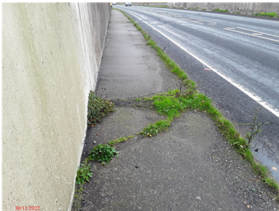
Span 3 - East Footway Footway cracked and sunk.
