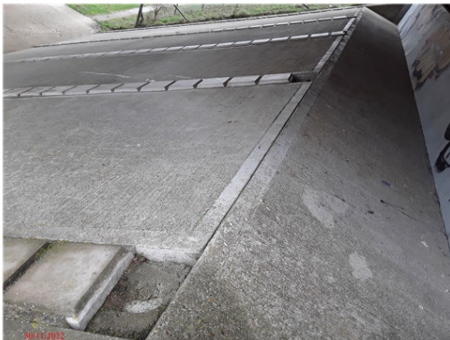
Span 3 - North East Revetment Missing revetment pavers
