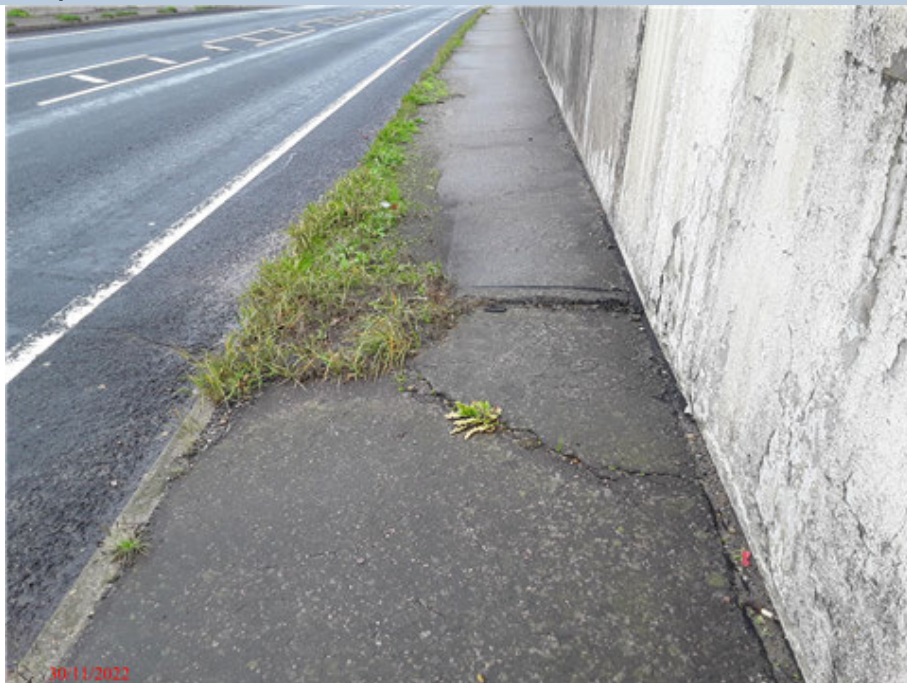
Span 1 - East Footway Footway cracked and sunk
