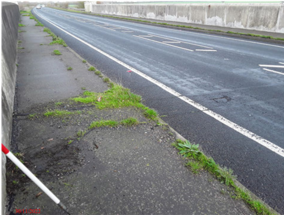
Span 1 - South West Footway Vegetation build up around APJ on footway.
