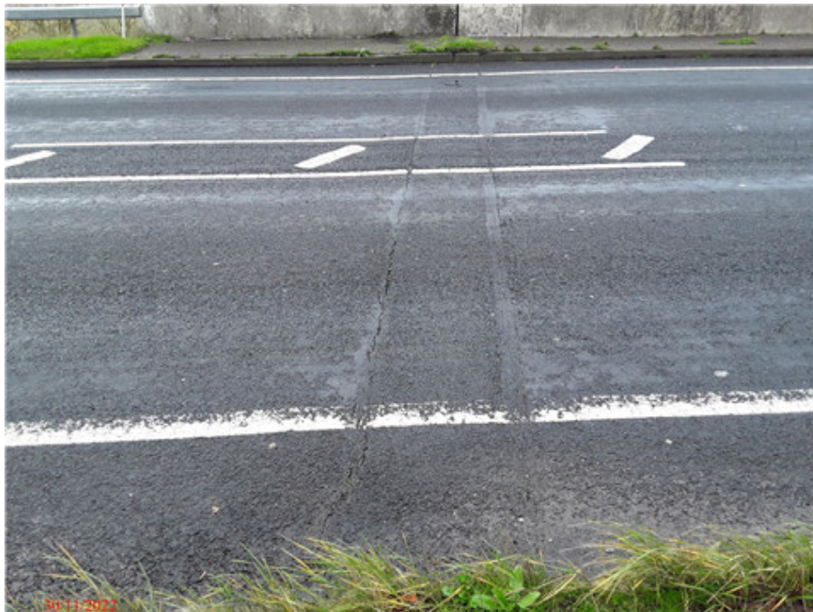
Span 1 - East Carriageway Cracks along APJ edges across carriageway
