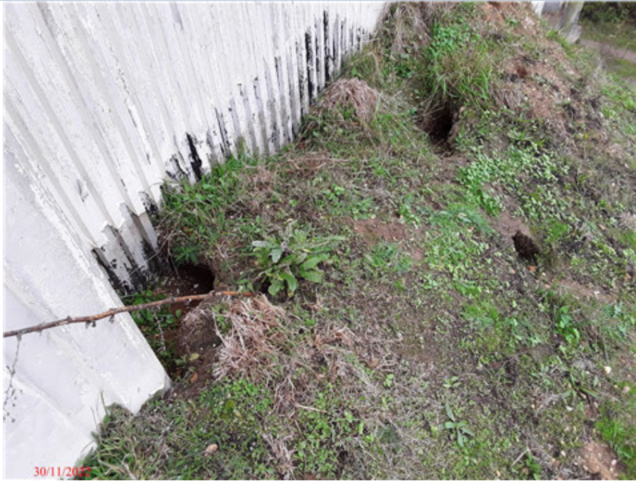
Span 3 - North West Embankment Animal habitat undermining elements.
