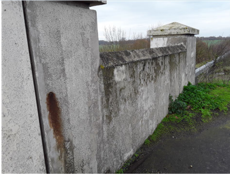
Span 3 - West Pilasters Protective paint top coat failing.
