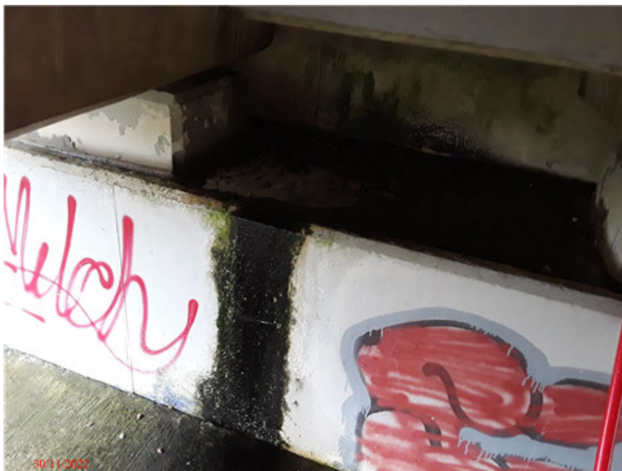
Span 1 - South East Abutment Staining to elements
