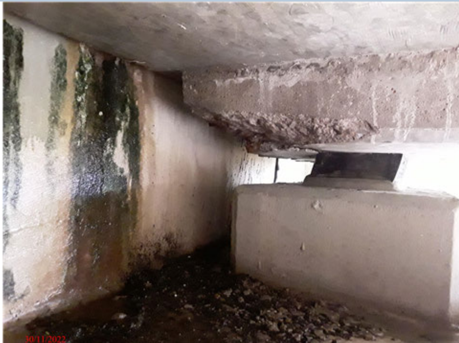
Span 1 - South West Deck Concrete spalling deck underside.
