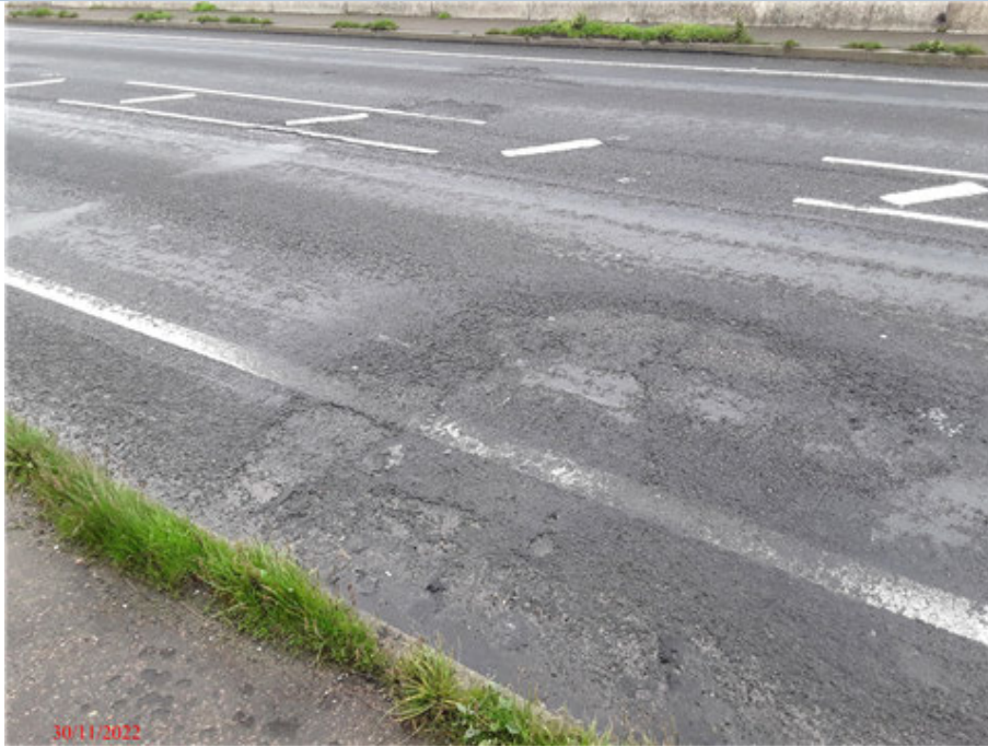
Span 2 - East Carriageway Patches of carriageway erosion across both lanes.
