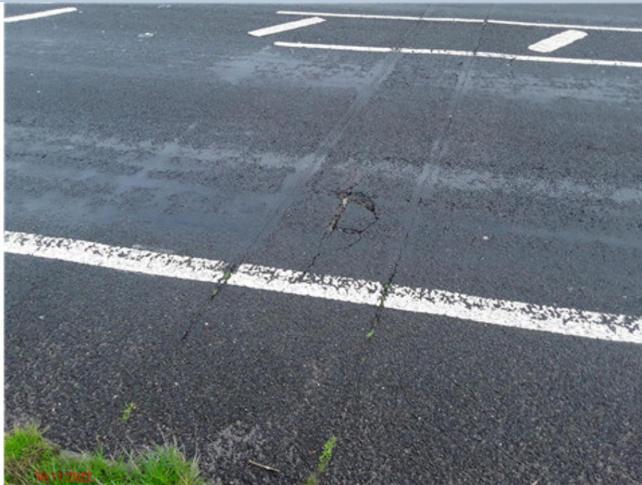
Span 1 - West Carriageway Surfacing Asphalt breaking up in APJ
