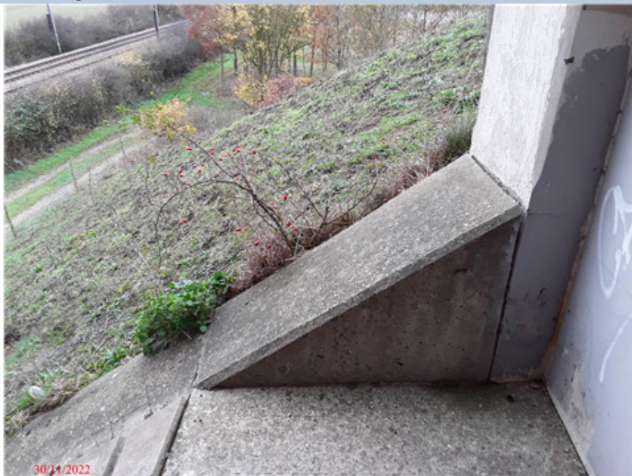
Span 3 - North West Buttress Separation of 15mm to pilaster
