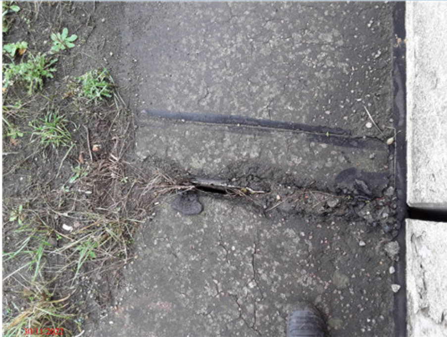
Span 1 - East Footway APJ Sealant debonded and missing
