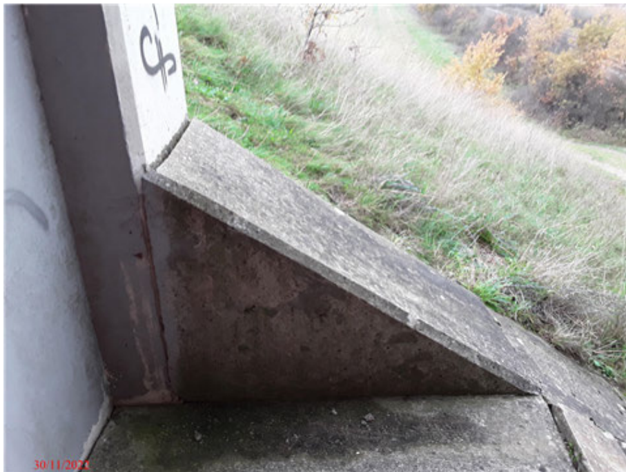
Span 1 - West Buttress Minor rotation to buttress.
