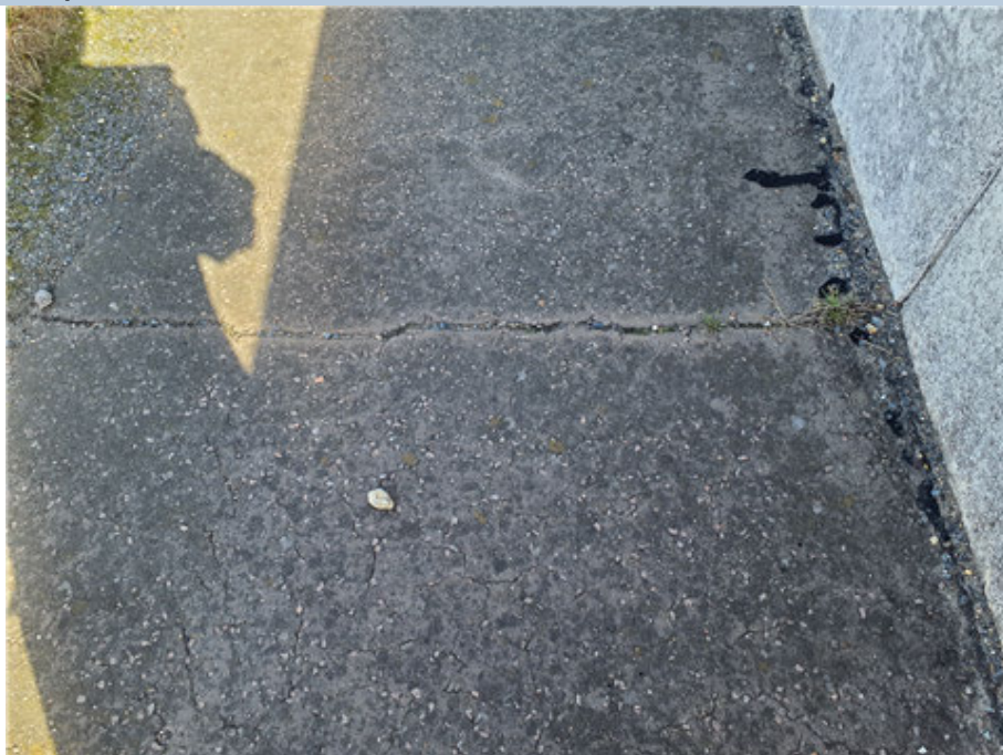
Easter footway Transverse crack and general crazing to footway.
