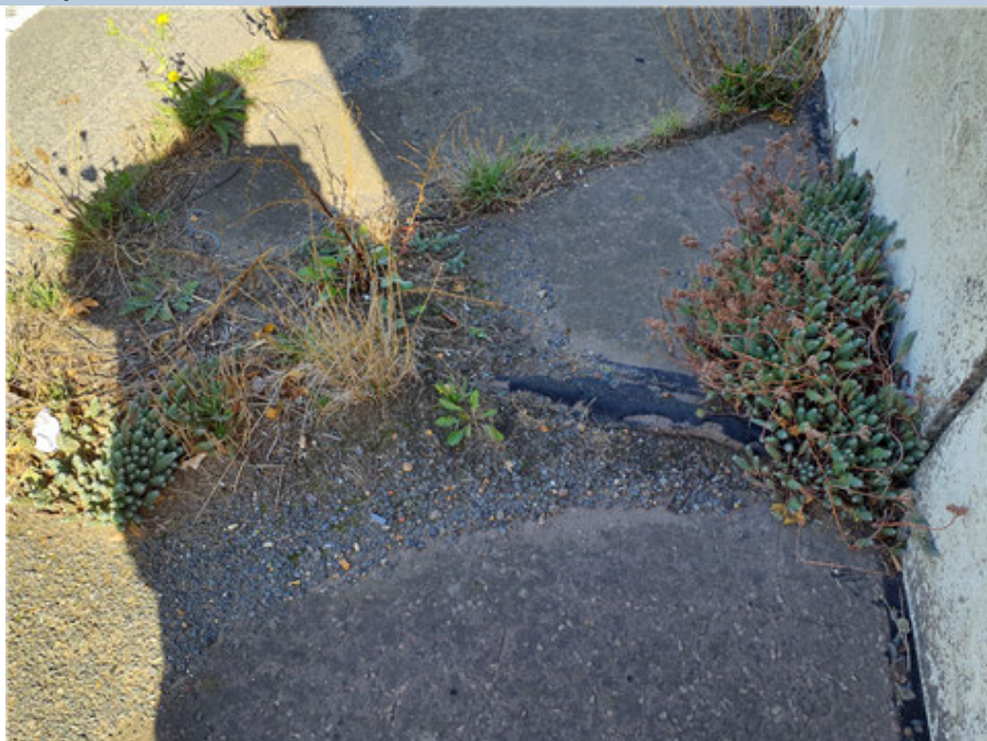
Eastern footway Transverse crack adjacent to deck joint with significant vegetation growth.
