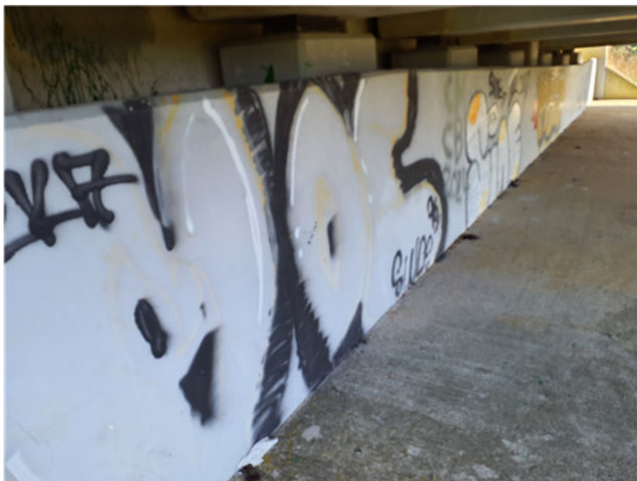
North abutment Non-offensive graffiti within view of the railway beneath span 2.
