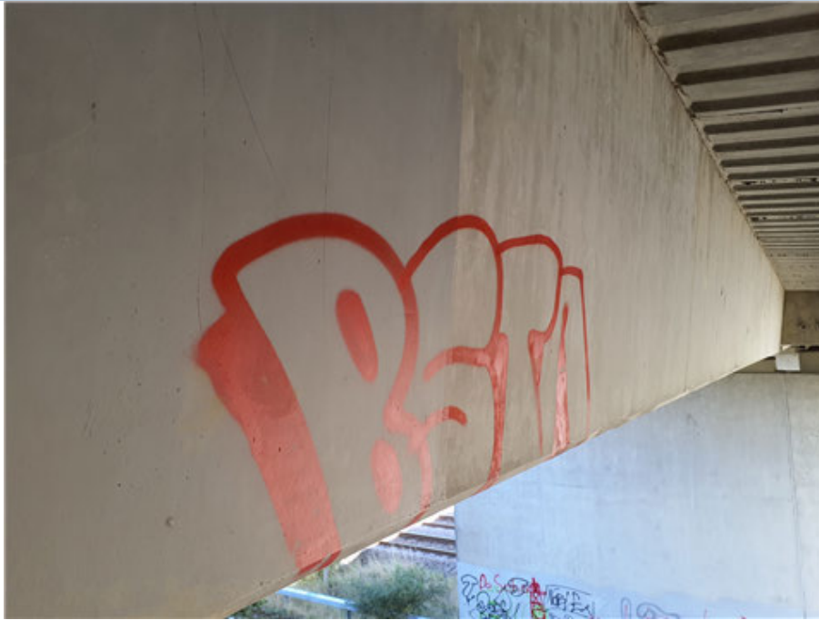
Main beam of span 1 Area of non-offensive spray paint graffiti to main beam.
