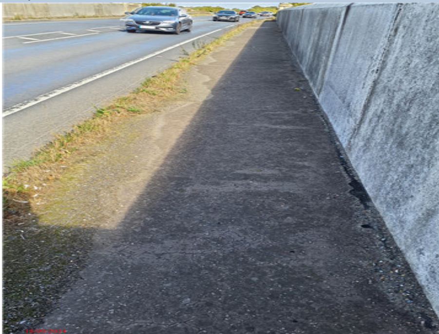
20240917_104040.jpg Vegetation growth to western kerb line
