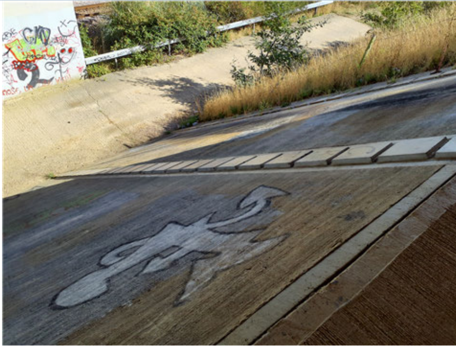
Revetment beneath span 1 Non-offensive graffiti to the revetment
