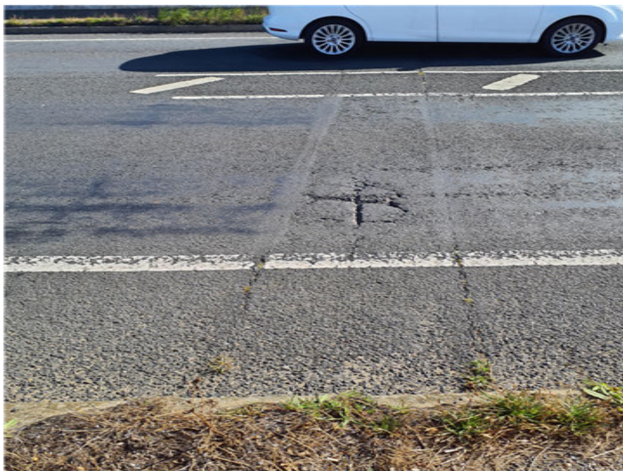
Eastern side of carriageway Cracking to surfacing over buried joint
