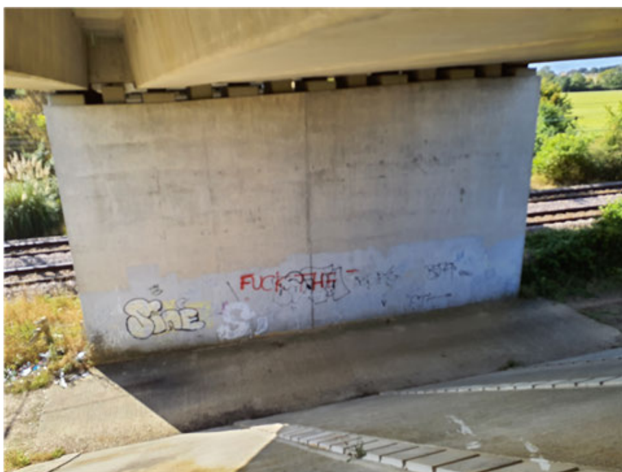
Substructure finish to pier 2 Area of offensive graffiti out of view of general public.
