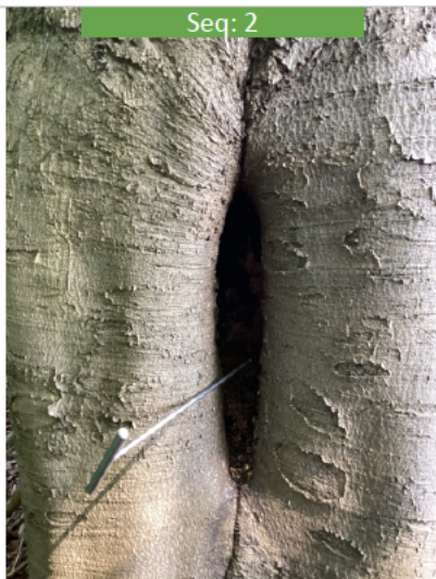
30/06/2025: Trunk - Trunk cavity
